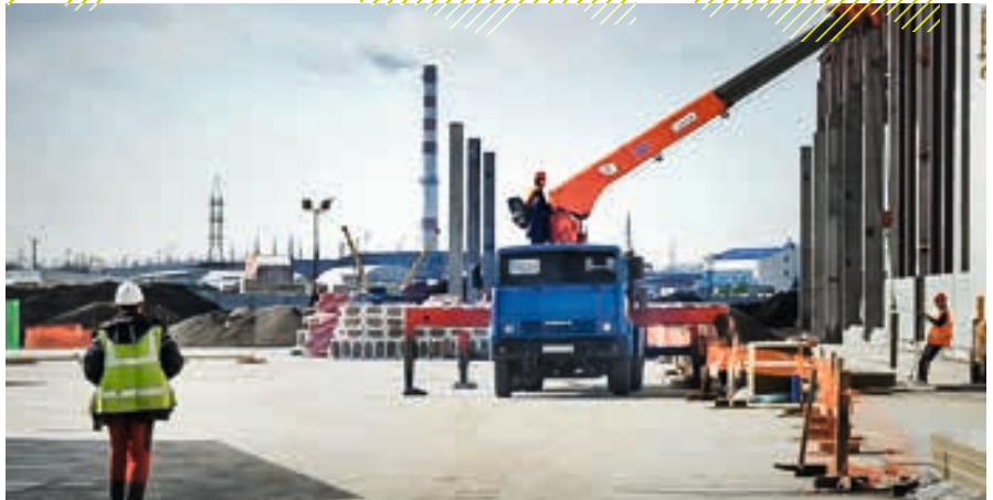
The expansion of the CLAAS factory in Krasnodar, Russia, is making good progress.
